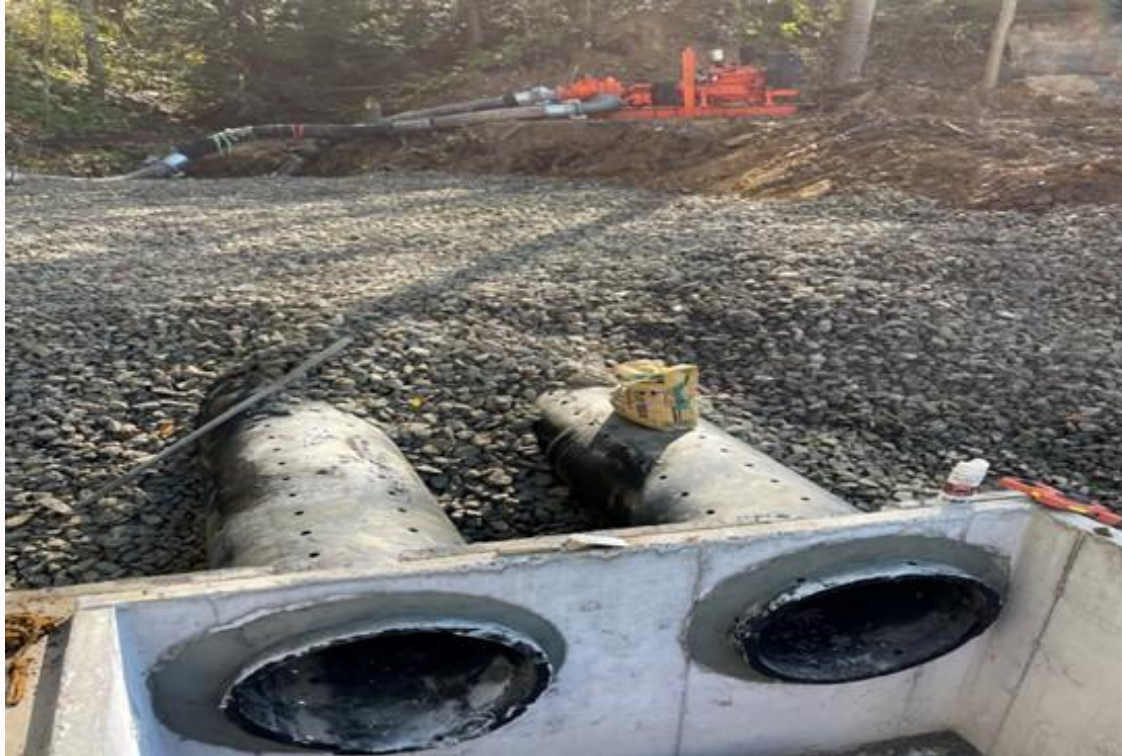
Mine Drain Collection System Two, 10-Inch PVC Pipes; Depth = 240 feet
