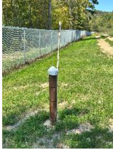
Standard steel guard setup w/ antenna extender
