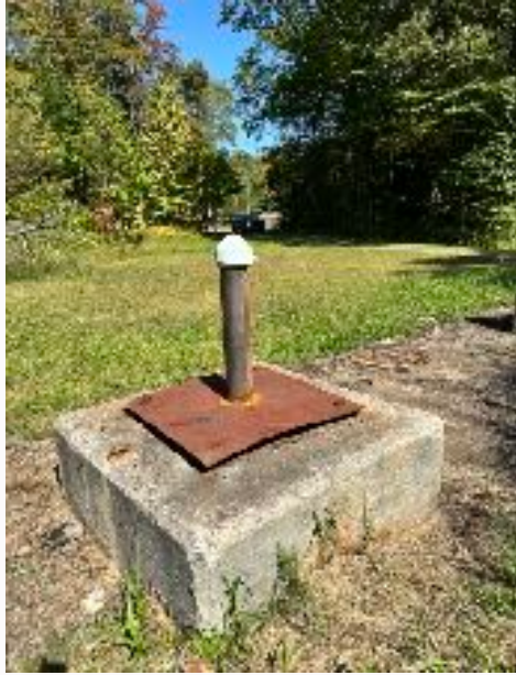
Logger on reinforced injection pad
