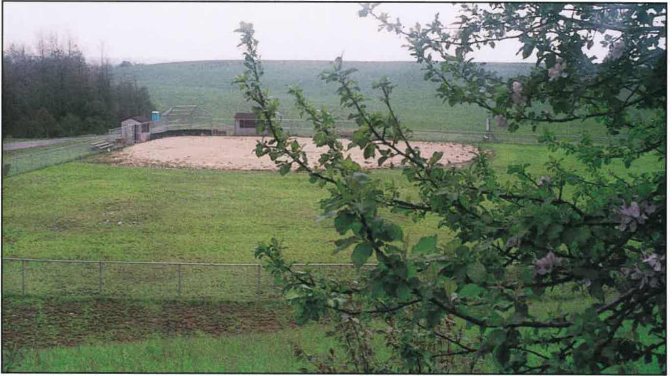
Buffalo went the extra mile to prepare this site near Thomas for ball field construction.
